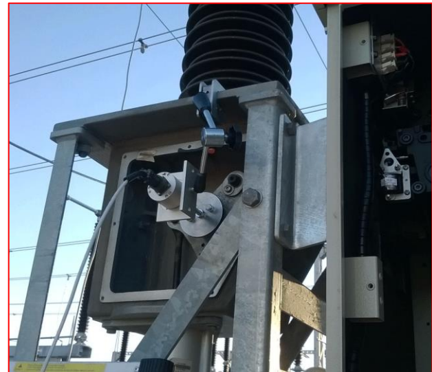
Figure 3-12: Digital rotary transducer mounted on ABB LTB 245 kV SF6 circuit breaker
