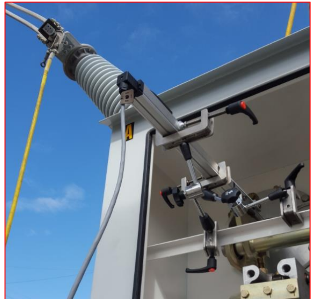
Figure 3-10: Analog linear transducer mounted on Mitsubishi SF6 138 kV 120-SFMP-40HE
